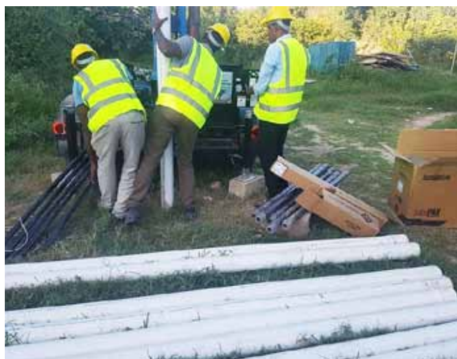
Installation of solar wells to provide the community with easy access to clean water (equipment/materials provided by Boswellness)
